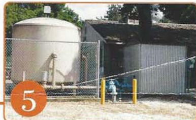
5 Investigate the feasibility of restoring the back up well for water supply
